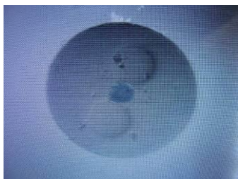
Damaged: Replacement required
