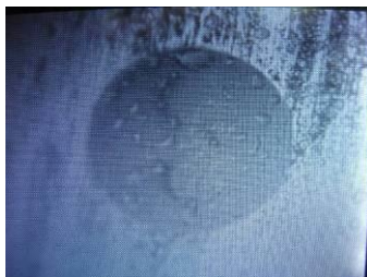
Dirty: Cleaning required
